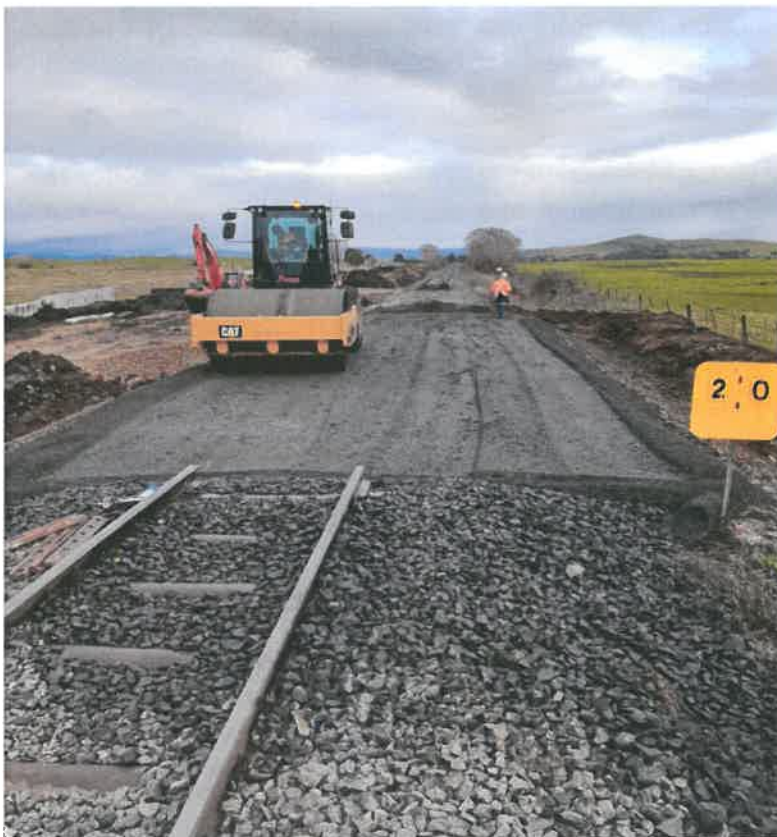
Formation work near Ross: TasRail is now delivering Tranche Two ($119.6 million) of the $376 million Tasmanian Freight Rail Revitalisation Program.
