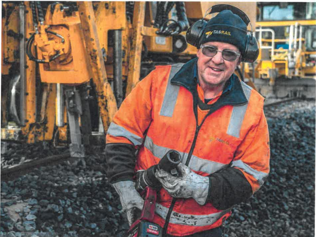
TasRail's Infrastructure team – operating the track tamper machine to ensure safe train operations
